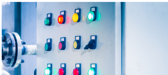
Electrical Panel Cabinet
